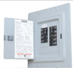
Electrical (Fuse Box)
